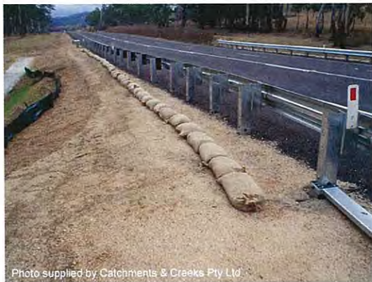
Photo 3 – Flow diversion berm used to minimise road runoff flowing down a steep, unstable section of the embankment
