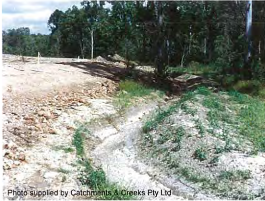
Photo 1 – Temporary diversion channel collecting 'dirty' water down-slope of a soil disturbance
