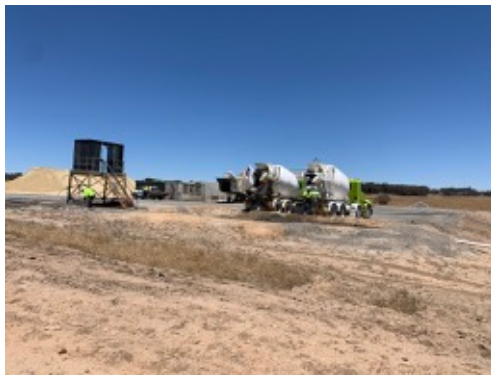
Photo 40: Concrete washout at batch plant.
