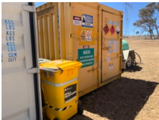
Photo 35: Substance storage container at TransGrid substation.
