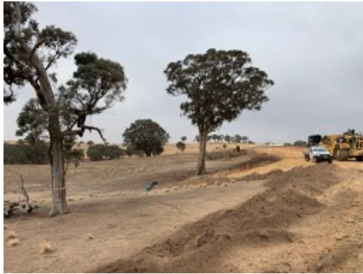
Photo 19: Example of project civil works for access tracks. Trees to be retained are marked, sediment fencing in drainage channel and top soil retained in wind row for rehabilitation purposes.
