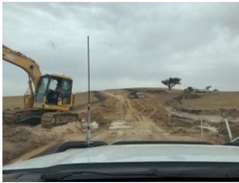
Photo 14: Access track 14 under construction. Top soil wind row for reuse and supporting erosion and sediment control.
