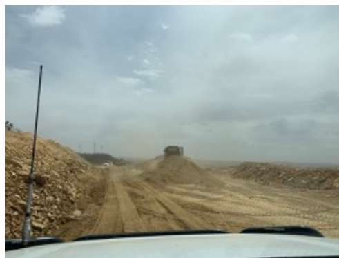
Photo 24: Location of crusher at WTG 3. Note dust storm beginning to impact site. Crushing activities had ceased due to winds. Water cart at location to suppress dust.
