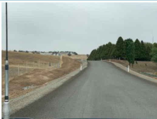
Photo 11: Example of road condition along Lerida Road South, including rock checks within drains.
