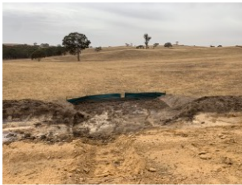
Photo 16: Example of site wide top soil wind row for reuse and supporting erosion and sediment control fence in key drainage points.
