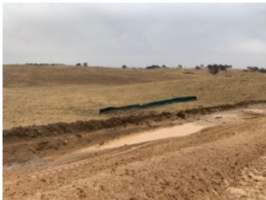
Photo 15: Example of site wide top soil wind row for reuse and supporting erosion and sediment control fence in key drainage points.
