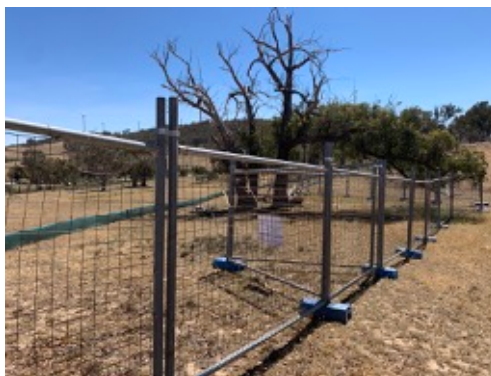
Photo 36: TransGrid substation perimeter fencing, RATCH installed sediment fence.
