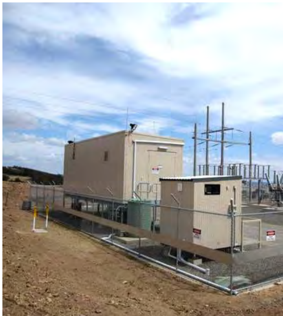
Plate 7 – Typical wind farm substation
