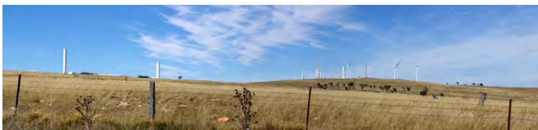
Plate 9 - Illustrating general construction activities at the Capital Wind Farm site, including views toward cranes, partial construction of towers and laydown areas.
