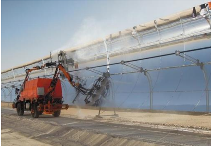
Figure 13. The cleaning system in Shams 1 CSP plant (29)
